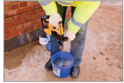
3. Stir thoroughly using a power-driven paddle mixer. Do not attempt to mix by hand as this will result in inadequate mixing
