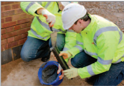
4. Check the piston is a snug fit in the cartridge and adjust in accordance with the pointing gun instructions. Load the mixture into the cartridge in the pointing gun immediately after agitating
